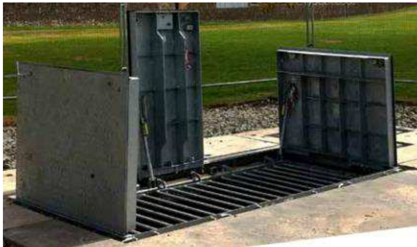
Figure 2-2 Surface Access covers
